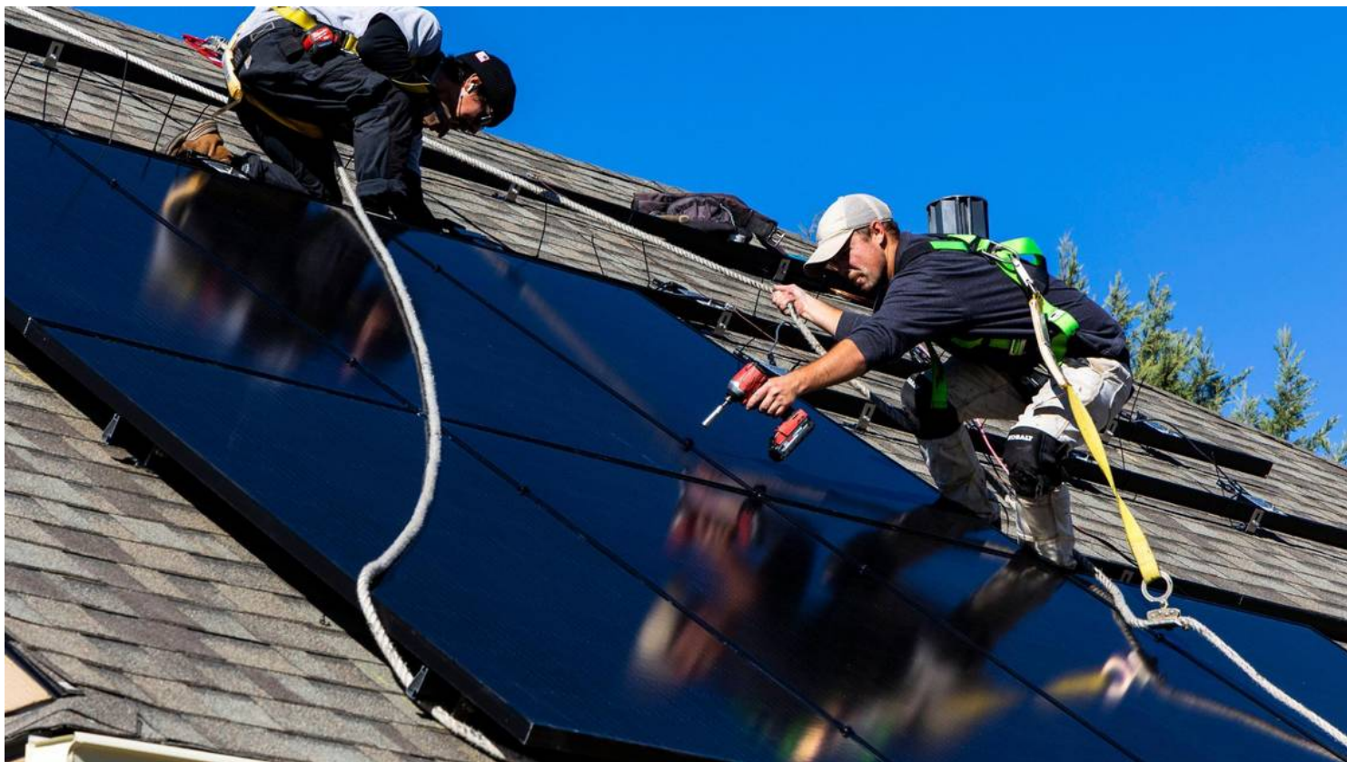
Sun Driven Solar employees Alec Carson, right, and Cesar Acuna, left, install solar panels onto the roof of Bob Kennedy's Nampa home in November. Darin Oswald doswald@idahostatesman.com
