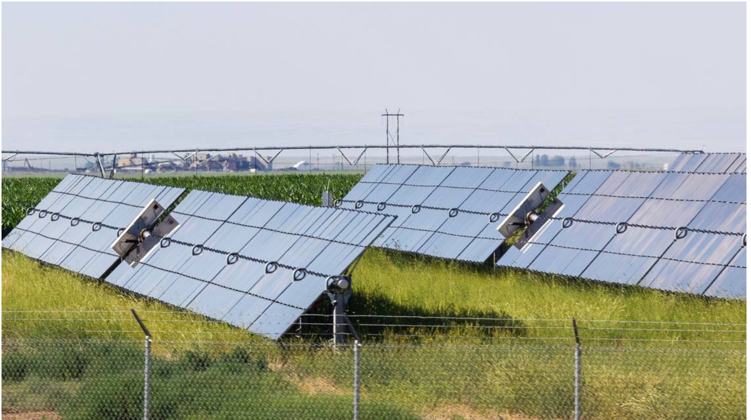
Solar panels seen near the highway between Boise and Mountain Home. Sarah Miller smiller@idahostatesman.com
