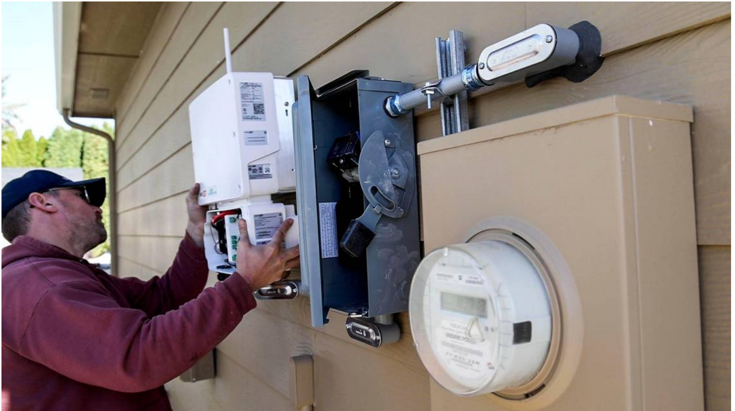
Electrician Matthew Jones, Electric Now, installs an inverter next to a power utility meter during a solar panel installation in Nampa in November. Darin Oswald doswald@idahostatesman.com
